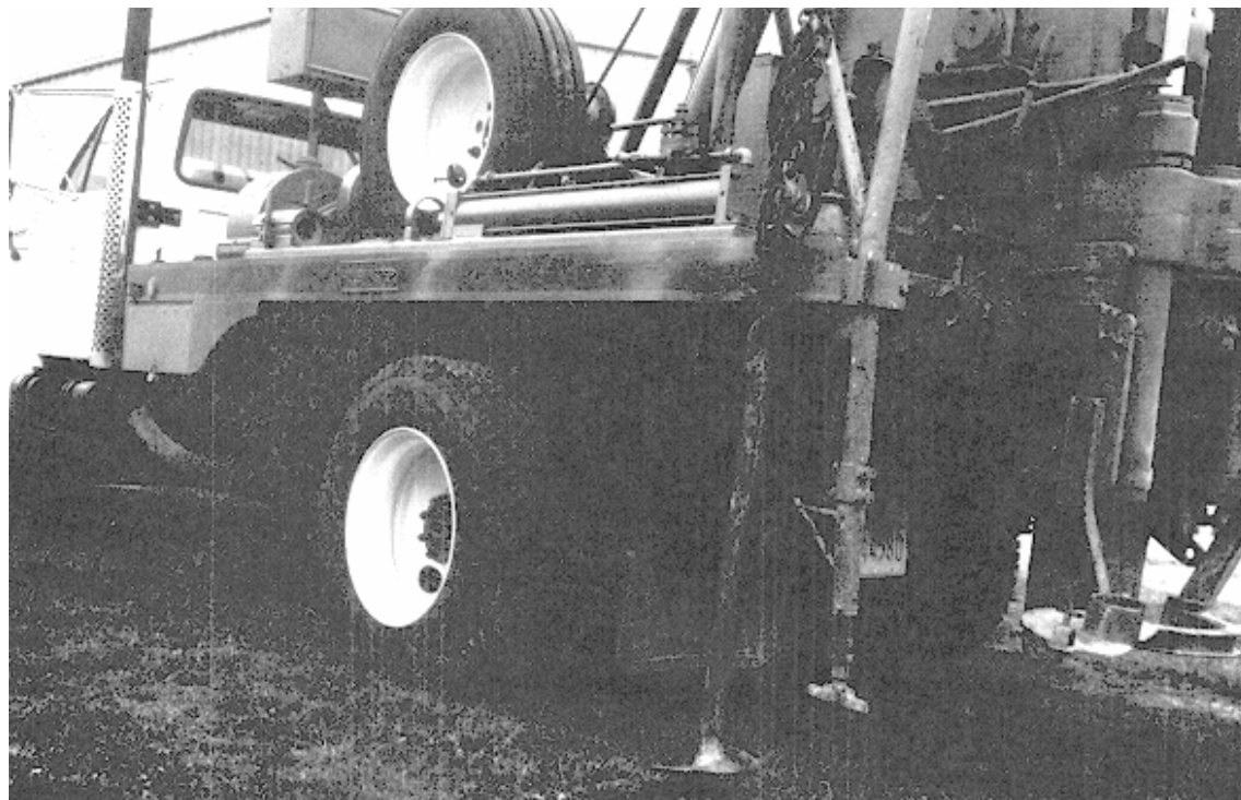
Figure 6-2. Photograph of screw-type earth anchors fastened to the drill rig with load binders to anchor the rig
